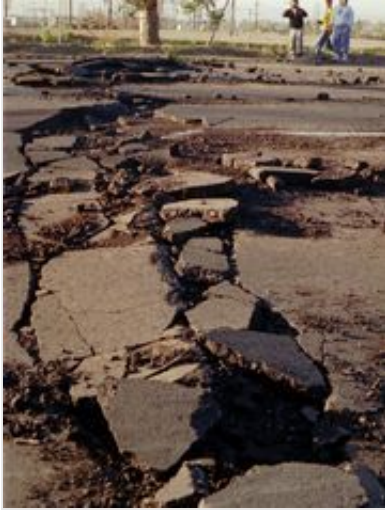
A section of San Fernando Boulevard in Sylmar, Calif., had a transversing thrust crack in 1994, after a major earthquake rocked Southern California. (Photo: William Wilson Lewis, AP)
